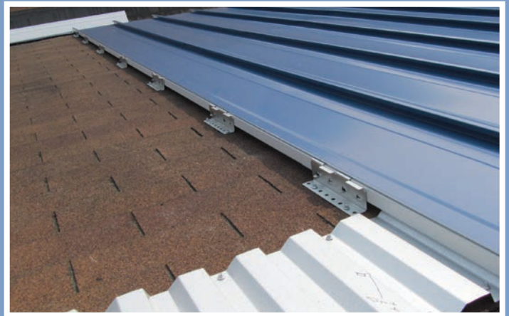
Corrugated sheeting installed at the ridge allows for continuous air flow between the existing and new roof while providing support for the panel and closure.
