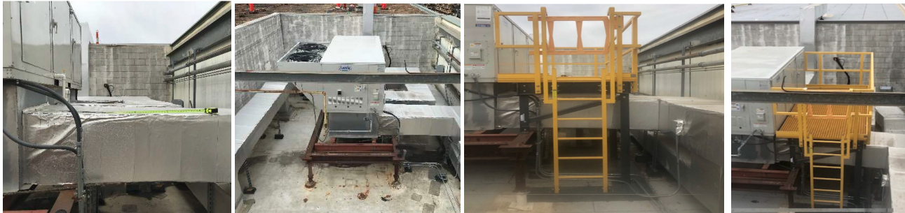
These photos show the extent of damage to the duct work
