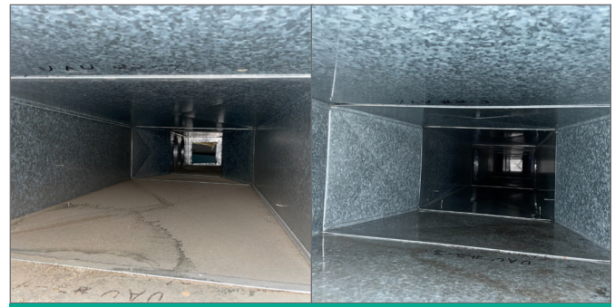
Ducts before PURE-Duct
